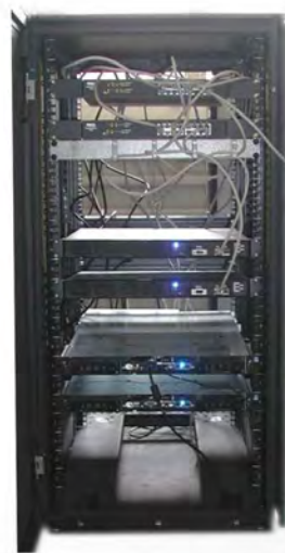
DELL SERVER RACK
